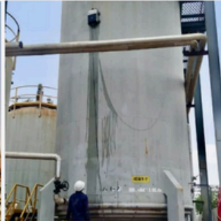
Storage Tanks - External
