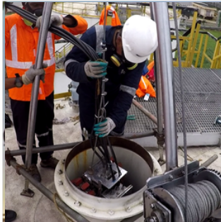
Storage Tanks - Internal
